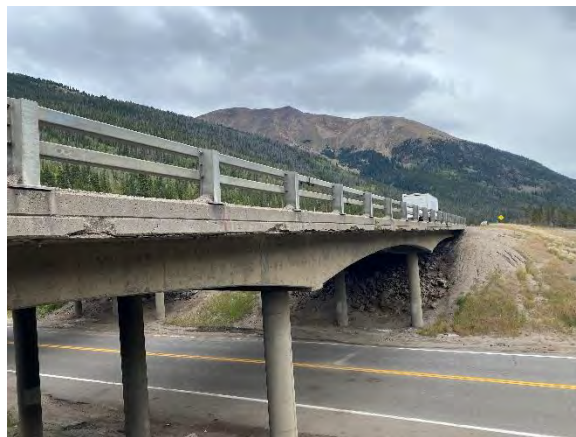
Figure 34. Typical spalling with exposed reinforcement at edges of deck
