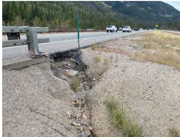
Figure 30. Erosion holes at ends of approach curbs
