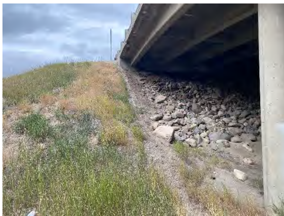
Figure 37. Erosion of berm embankments
