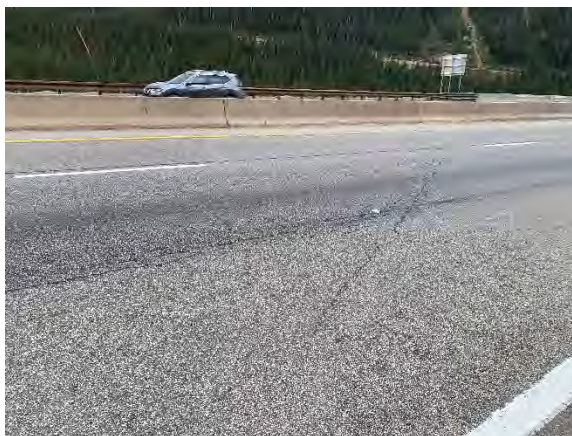
Figure 10. Transverse cracking of asphalt over Abutment 1
