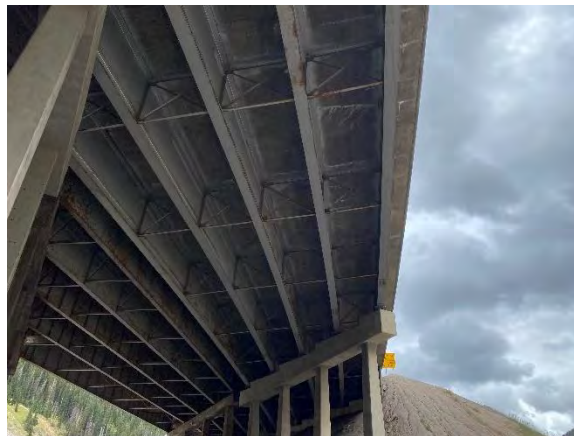
Figure 24. Typical view of underside of deck showing areas of cracking with efflorescence
