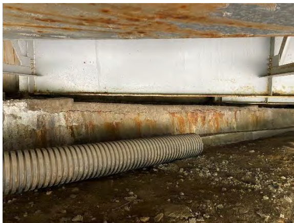
Figure 16. Delamination and rust staining on Abutment 1 girder seat
