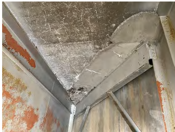
Figure 25. Cracking with efflorescence on underside of joint header at Abutment 4
