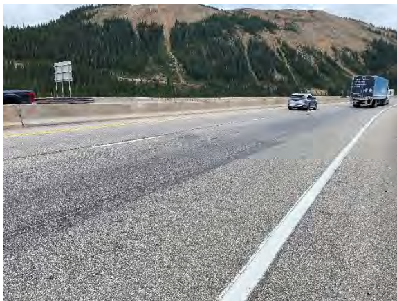
Figure 7. Asphalt patches in wearing surface
