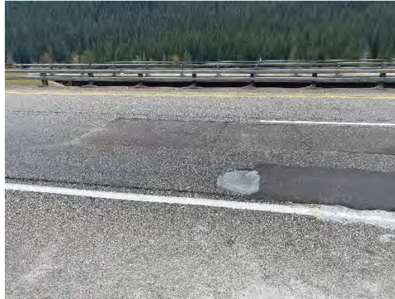
Figure 39. Asphalt patches in wearing surface
