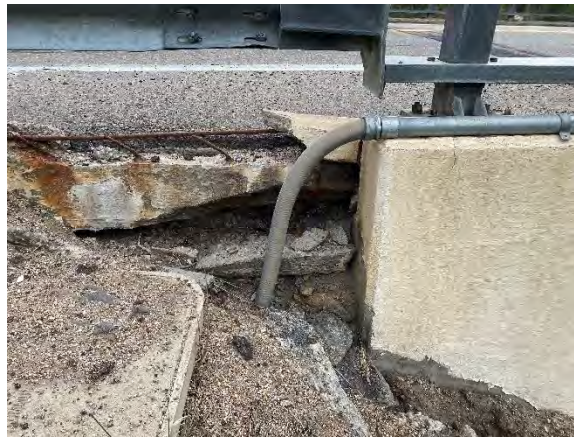
Figure 49. Typical undermining of approach slabs and damage to curbs on approach slabs. Right side of rear approach slab
