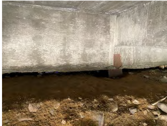
Figure 36. Off-center pile under Girder C at Abutment 1
