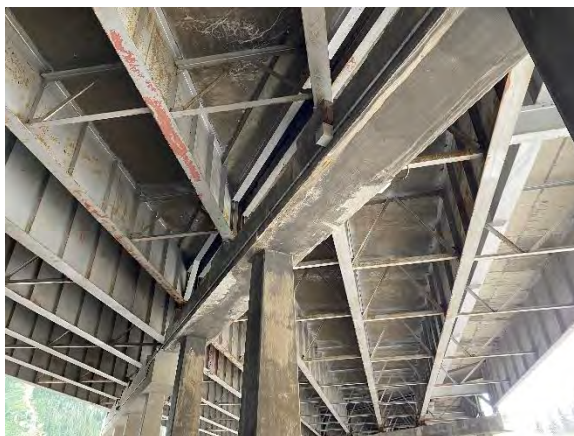
Figure 18. Failing, cracked patches on bottom edges of Pier 3
