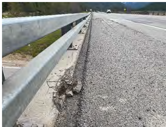
Figure 41. Delamination and spalls on the front face of the curbs
