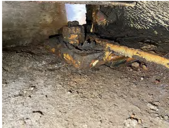
Figure 52. Crushing and bulging of bearing pad 3E
