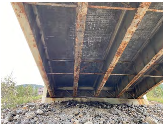
Figure 50. Typical view of underside of deck showing areas of cracking with efflorescence, Span 2 at Abutment 3
