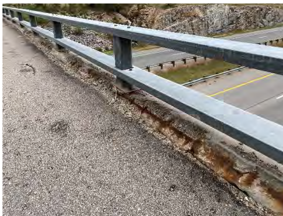
Figure 47. Typical spalls with exposed corroded reinforcement in curbs and “Type N” bridge rail
