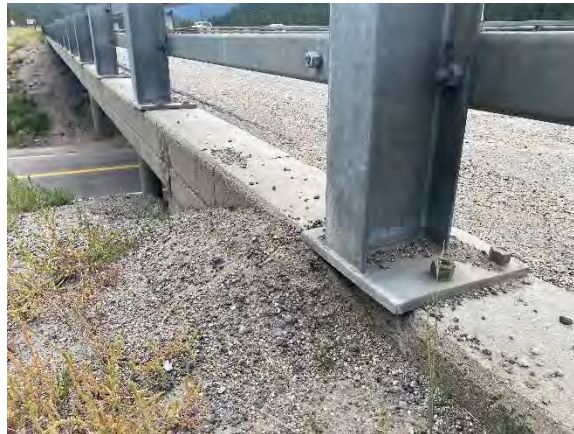
Figure 40. Disengaged nuts on bridge rail anchors
