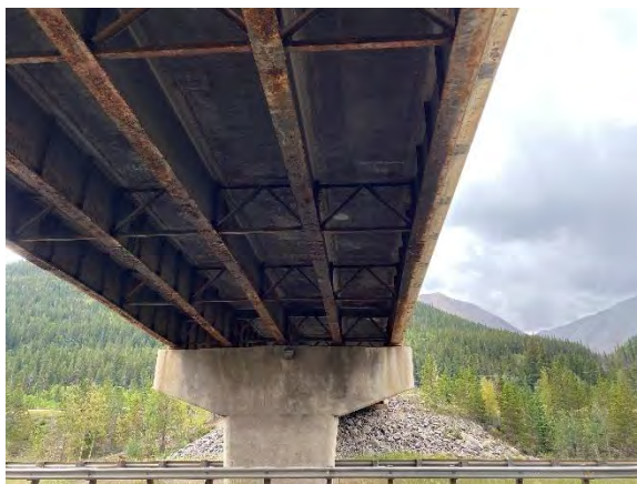
Figure 51. View showing general condition of superstructure paint and corrosion on girders
