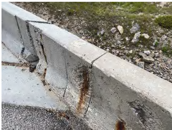
Figure 8. Typical deterioration of outside bridge rail
