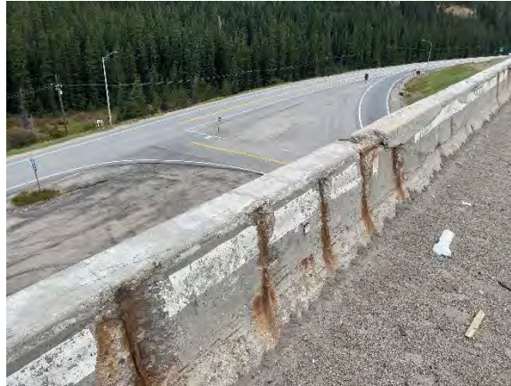
Figure 23. Typical spalling with exposed corroded reinforcement in the concrete barriers
