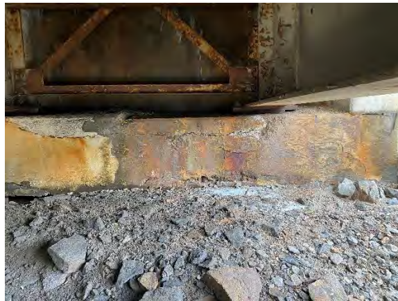
Figure 53. Typical delamination and rust staining on girder seats, Abutment 1 Bay A
