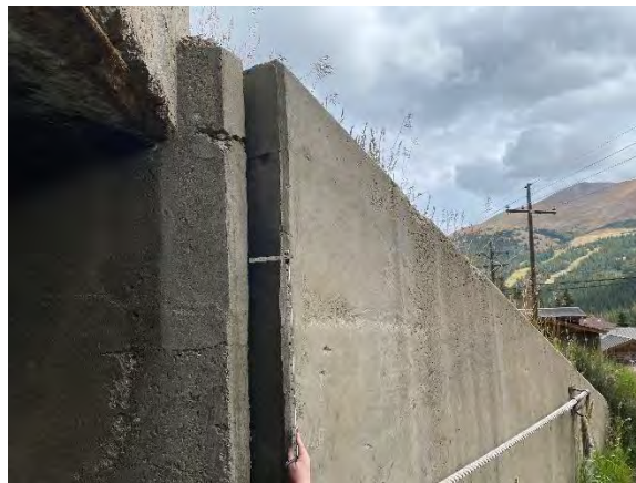
Figure 61. Leaning of southeast wingwall
