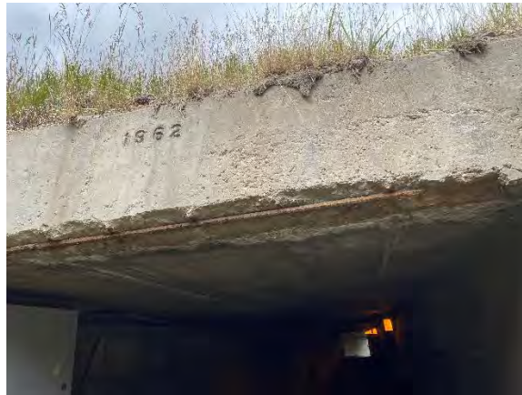
Figure 60. Spall with exposed rebar at outlet
