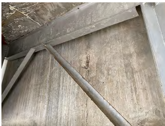
Figure 27. Spall with exposed reinforcement on Abutment 1, Bay D
