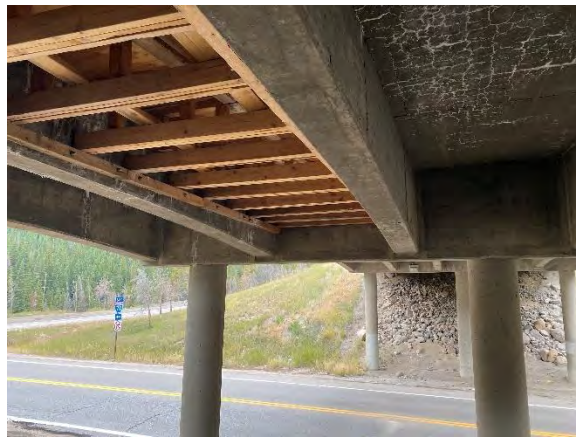
Figure 33. Permanent form work for concrete repair (Bay 3D) and map cracking with efflorescence (Bay 3C)
