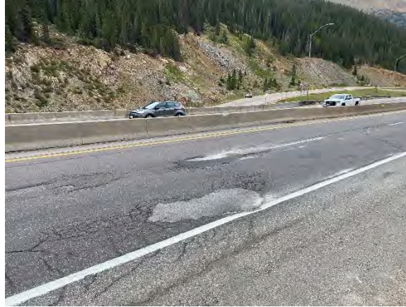
Figure 20. Typical potholes in asphalt wearing surface
