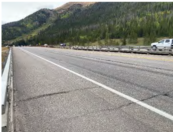
Figure 29. Asphalt rutting in driving lane
