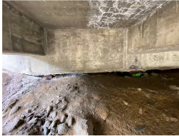
Figure 35. Exposed piles at Abutment 1
