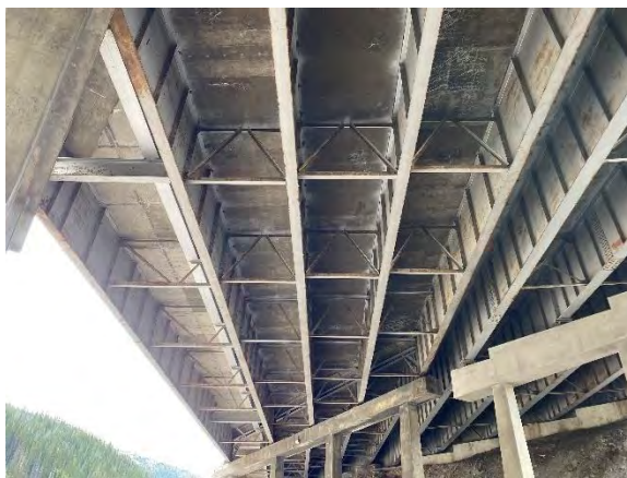
Figure 12. Typical view of underside of deck showing areas of patch and cracking with efflorescence
