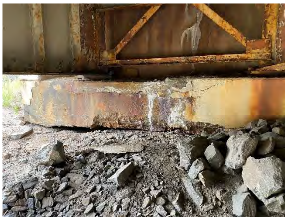
Figure 54. Failed patch exposing corroded reinforcement, Abutment 1 Bay D
