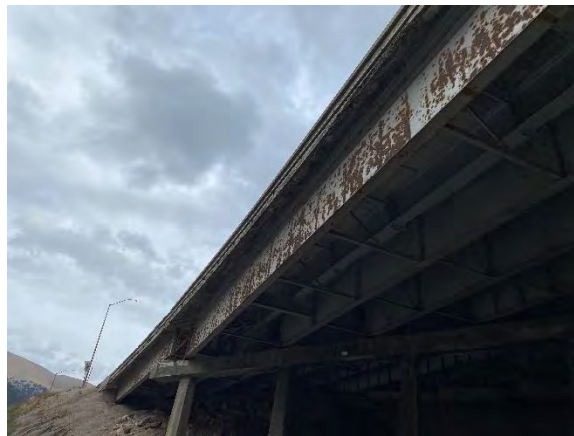
Figure 14. View showing general condition of superstructure paint and corrosion on girders
