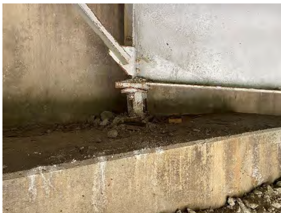
Figure 26. Typical condition of movable bearings, Abutment 1 Girder B
