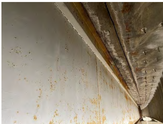
Figure 11. Drainage through longitudinal joint with F-13-P on to Girder E, corrosion on top flange of Girder E
