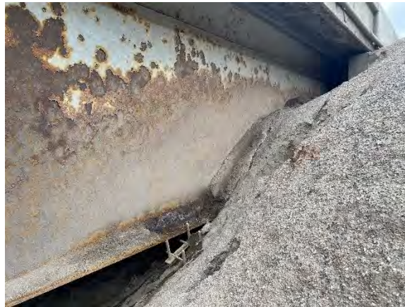
Figure 13. Debris on Girder 1A with uncovered area
